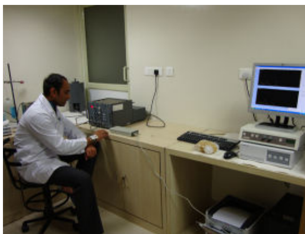
NaI Scintillation Detector (well type) based gamma ray spectroscopy system with 8k MCA, installed in QC lab of a medical cyclotron facility. System is used to test isotope purity & energy of the Radio-nuclides such as FDG / F-18 or Tc-99, I-131etc., produced
