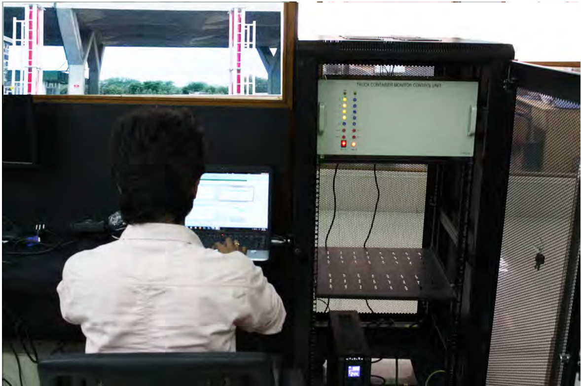
Data acquisition and alarm unit
