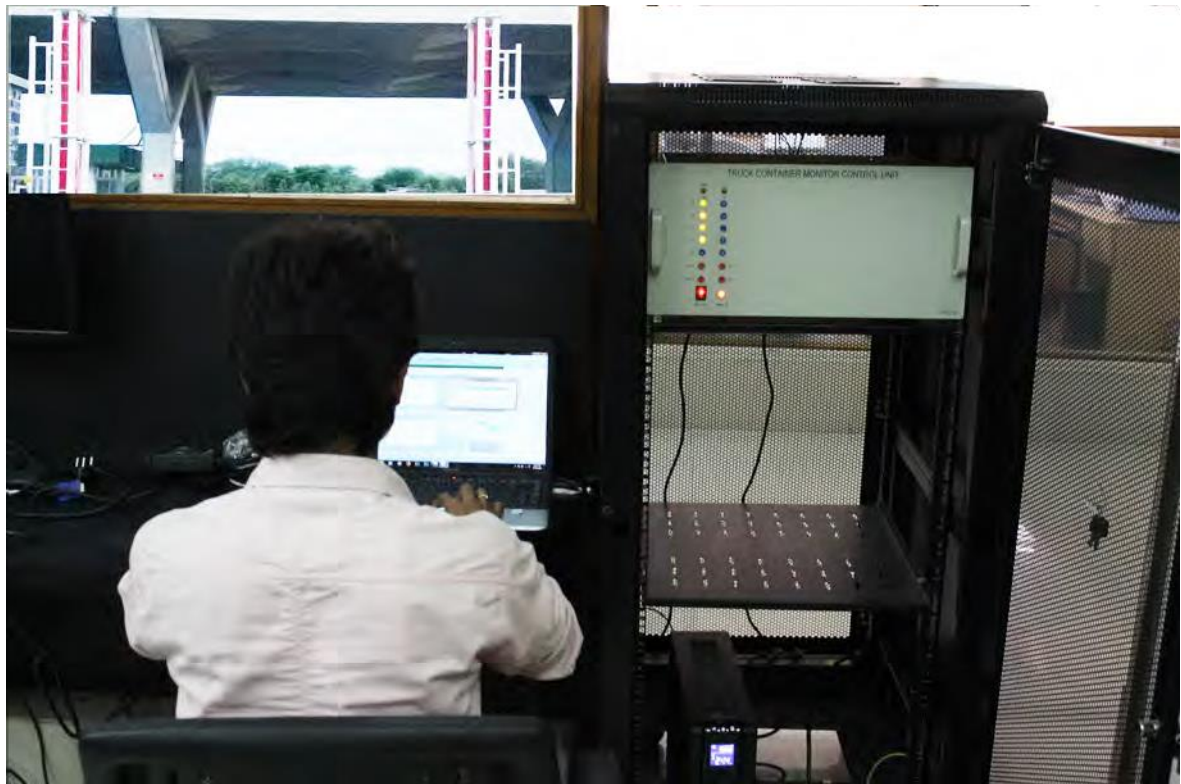
Data acquisition and alarm unit
